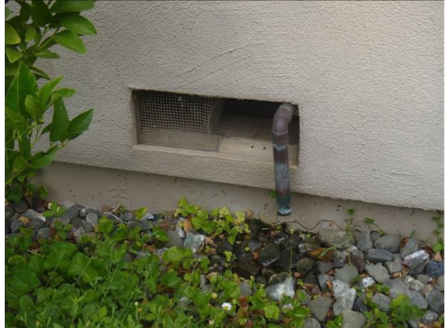
Structure Perimeter Exterior Vent Screens Attention
